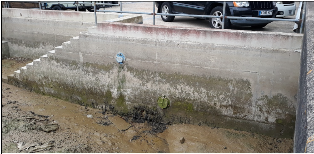
Flood gate to basement car park
